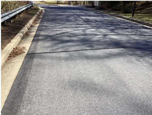
Asphalt pavement street overview - Note previous repairs
