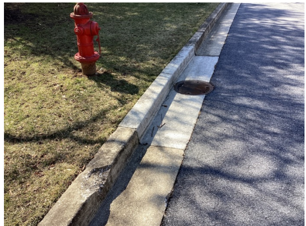
Previous repairs evident
