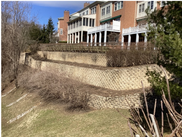
Masonry retaining walls overview - Note minor stains
