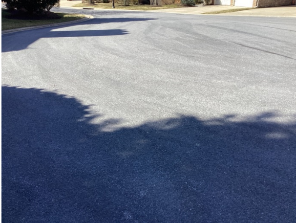
Asphalt pavement street overview - Note minor wear and previous cracks sealed
